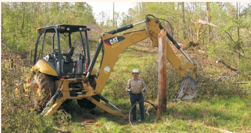
Crews worked around the clock to repair damage from the F-3 tornado that swept through the area April 16, 2011.
