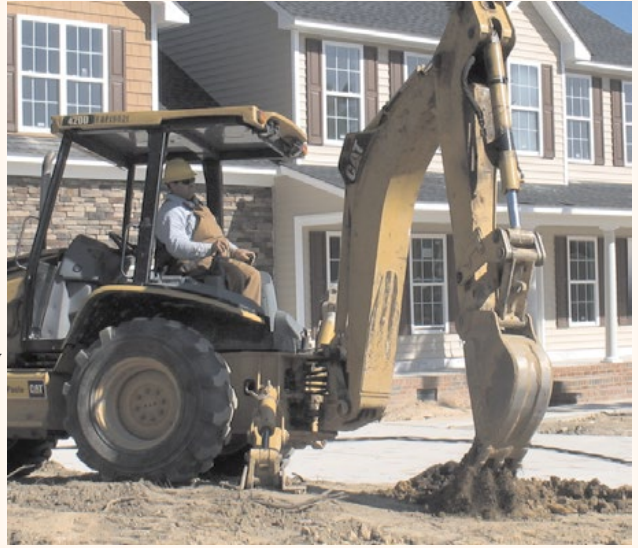
New housing developments contributed to the amount of underground service installed in 2011.
