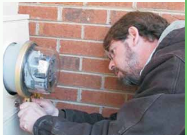
Victor Burns installs necessary meter equipment for a member to use the Pre-Pay Program.
